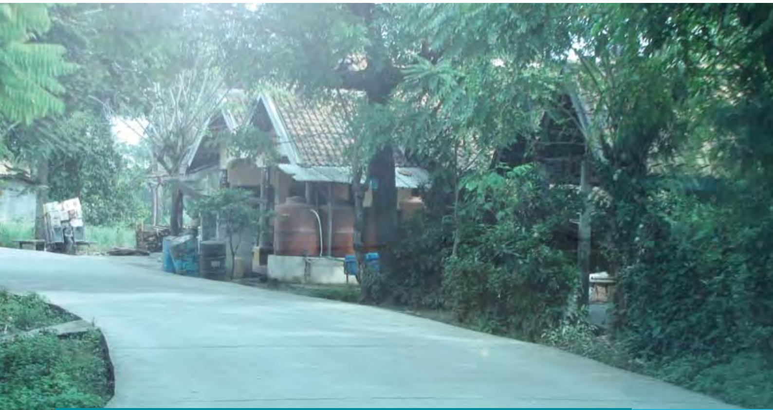
Program CSR Infrastruktur Pembetonan Jalan, Desa Muara Bakti Babelan / Concrete road CSR infrastructure program at Muara Bakti Babelan Village
